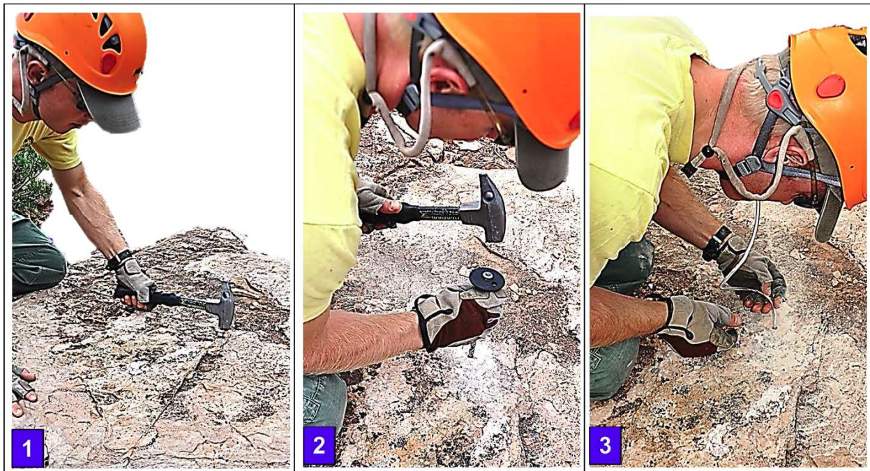
Figure 131- Bolting technique; 1.) Testing the placement site and clearing loose rock. 2.) Hand drilling with a twisting motion to a depth \frac{1}{2} inch deeper than the bolt being placed. 3.) Using a blow tube to remove rock dust and clear the hole prior to placement.
